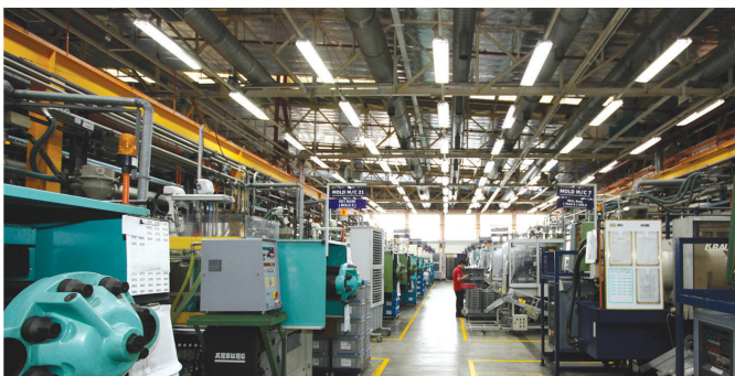
Meralco recommended replacing SMPI's fluorescent lights with LED bulbs at its production floors for better energy efficiency.
