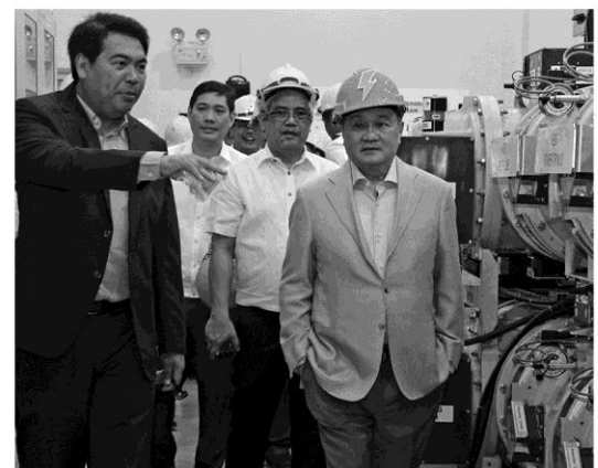
Meralco VP & Head of Sub-Transmission Services Antonio M. Abuel, Jr. (left) shows Meralco Chairman Manuel V. Pangilinan (right) around the facilities of PAGCOR-1 Sub-station.
